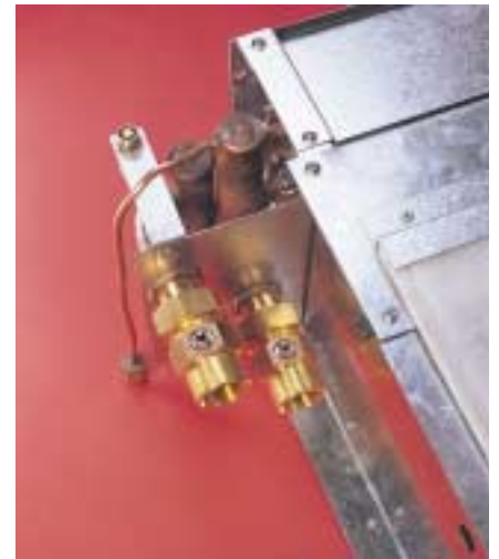
Fitted isolating ball valves
